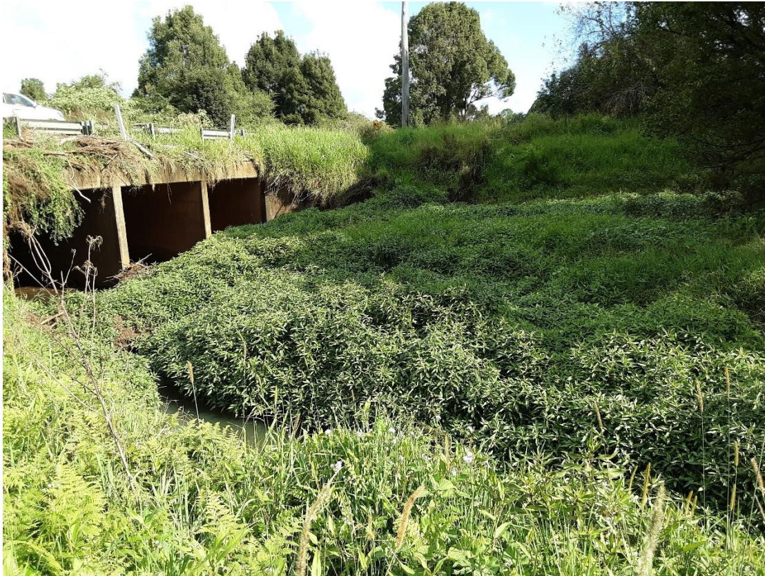
Figure 9: Colonisation of weeds in areas of built-up sediment such as near the Culverts under Lismore Road (looking south west)
